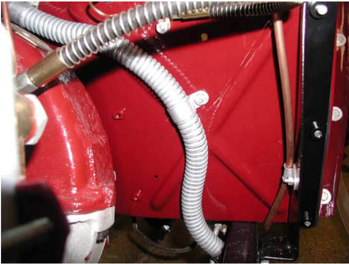
7 – Main conduit from frame
